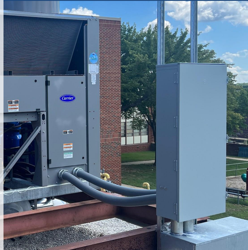
Thomas Stone ES (HVAC Replacement)
