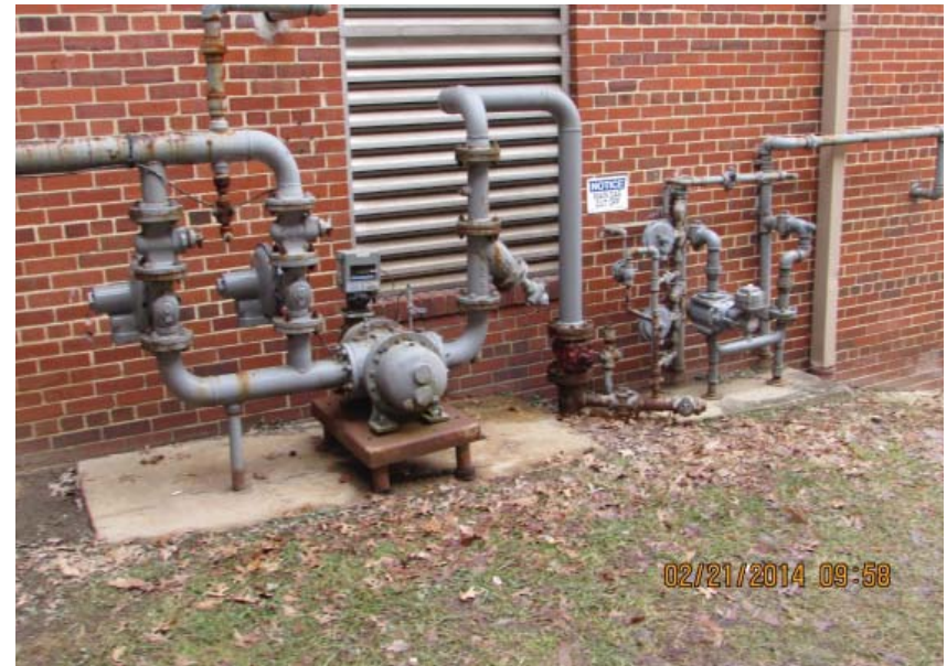
Incoming Gas Service
