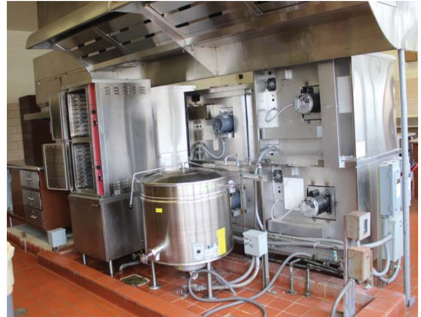
Existing Steam Side of the Cooking Line-Up
