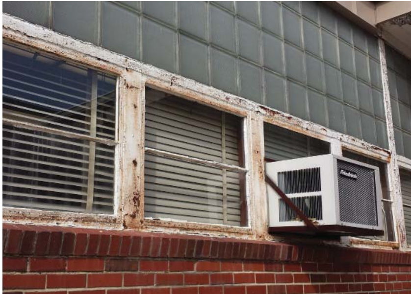
Existing windows exhibit significant deterioration
