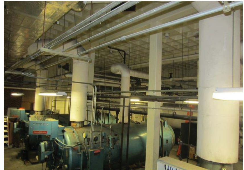
also provide steam to a steam-to-hot water converter located in the second mechanical room which was built with the 1964 addition.
