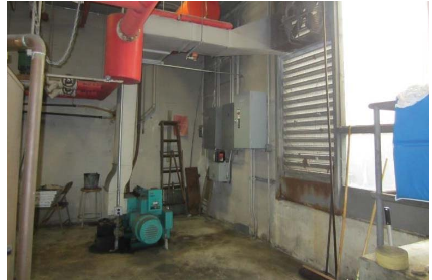
Life Safety Generator with Louver and Exhaust
