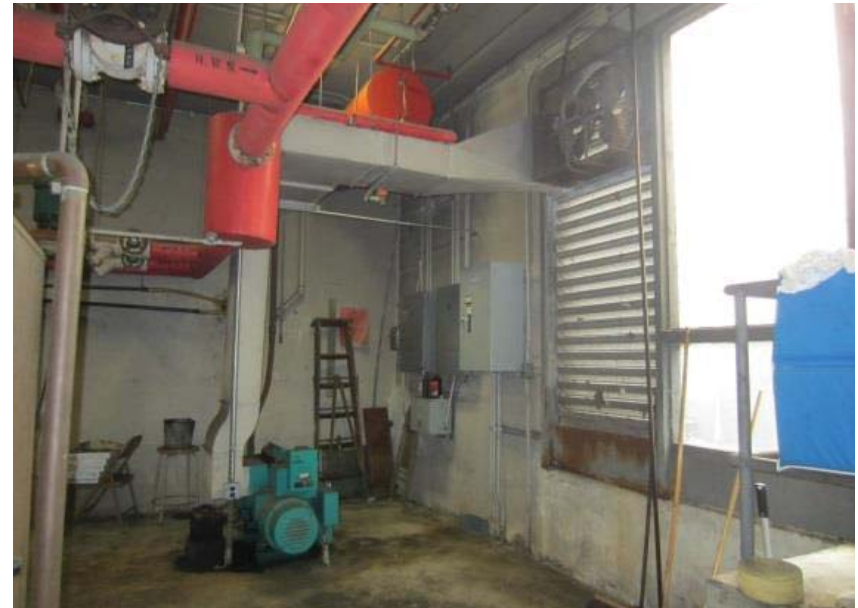
Generator in Auditorium for local life safety
