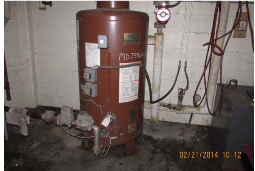
Gas Fired Domestic Water Heater
