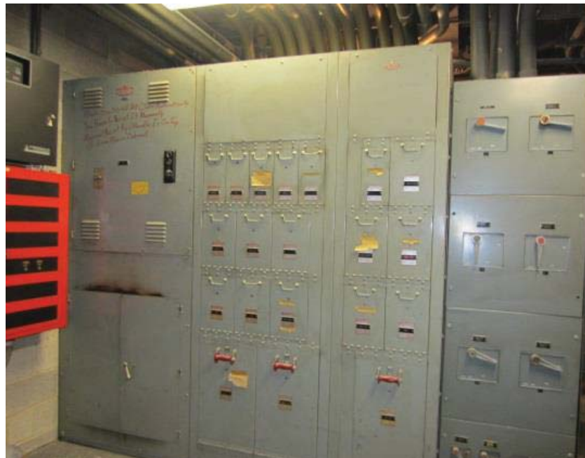
Original 208Y120 volt switchboard
