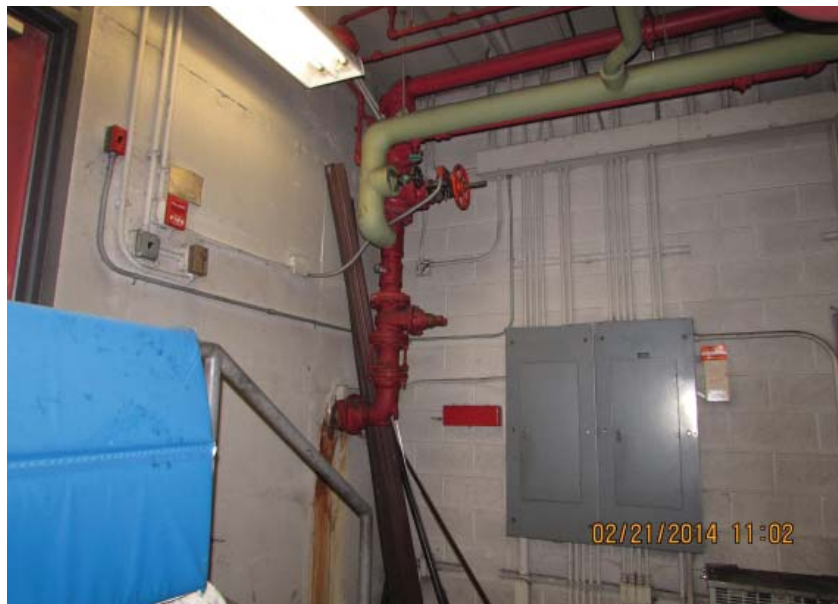
Incoming Water Service - Main Building
