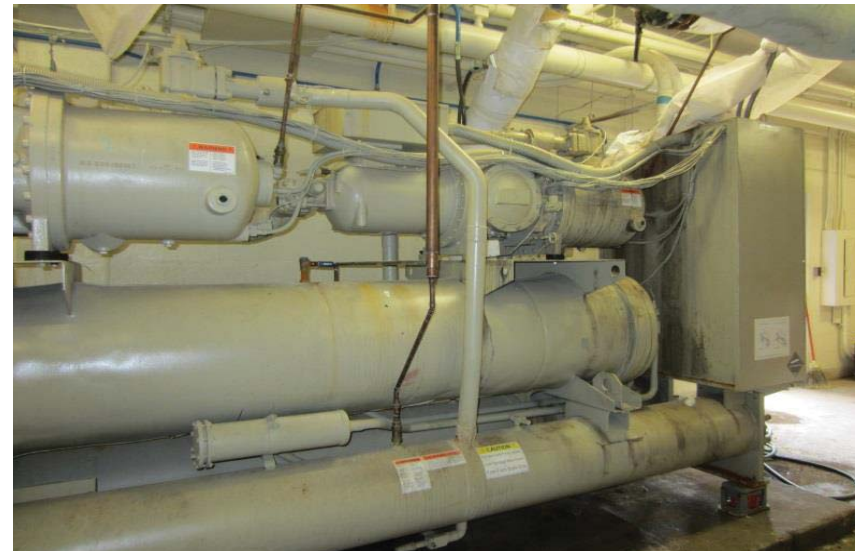
Water-Cooled Chiller #1 Mechanical Room
