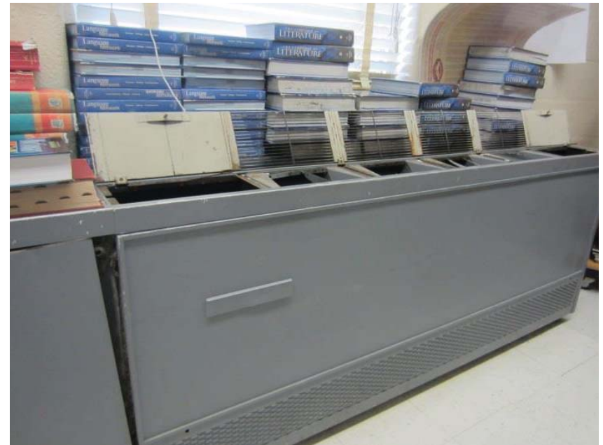
Typical Classroom in Post-1964 Buildings – Heating and Cooling Unit Ventilators via hot and chilled water coils
