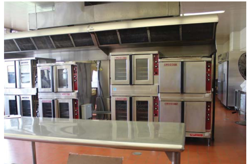
Existing banks of Double Stacked Convection Ovens
