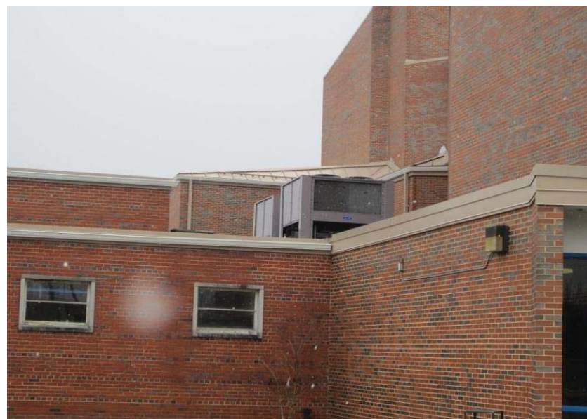
Air-Cooled Condensing Units on Roof Near Auditorium
