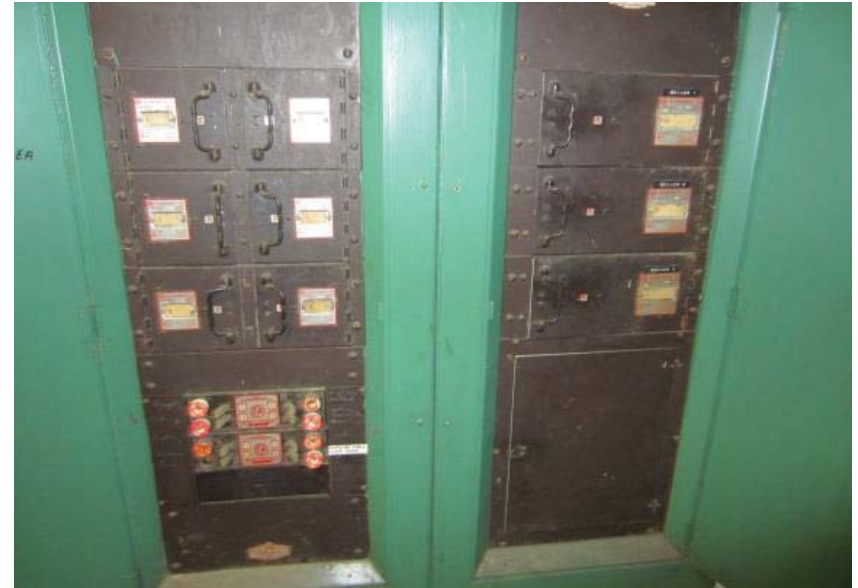
Older panelboard, typically unlabeled
