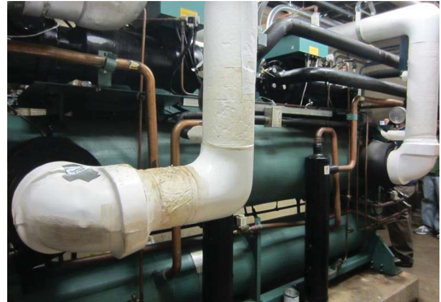
Water-Cooled Chiller #2 - Penthouse
