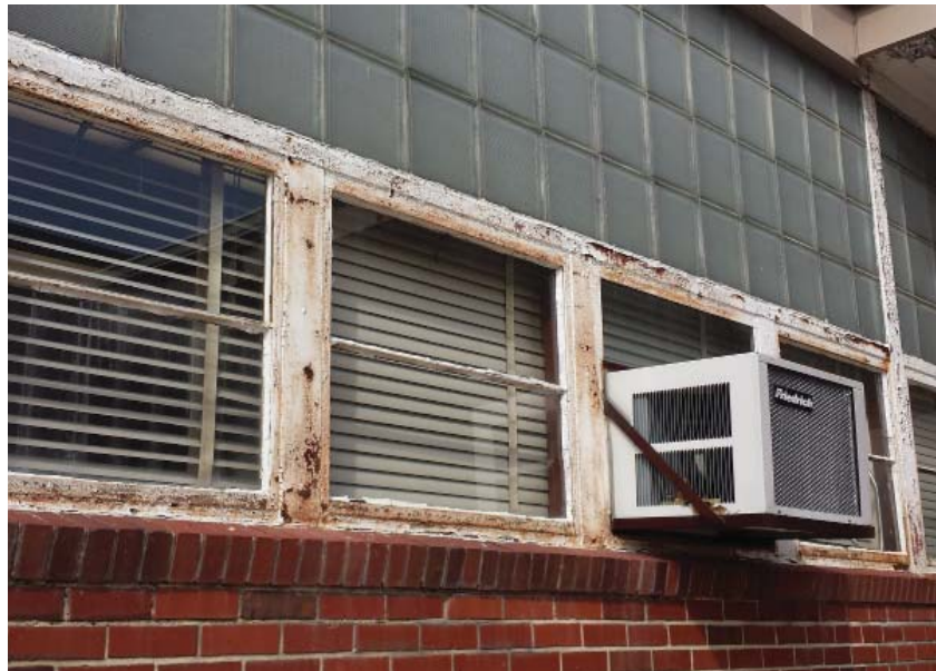
Existing windows exhibit significant deterioration
