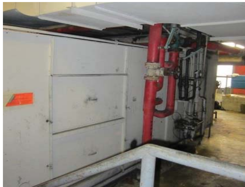
Air Handler – Serving the Auditorium
