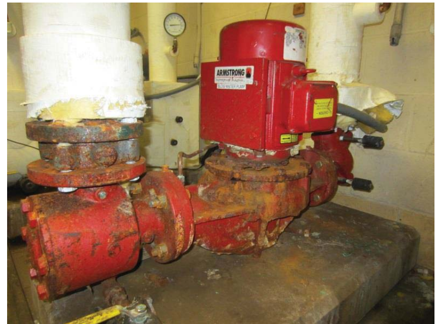
Corroded Base- Mounted Pump
