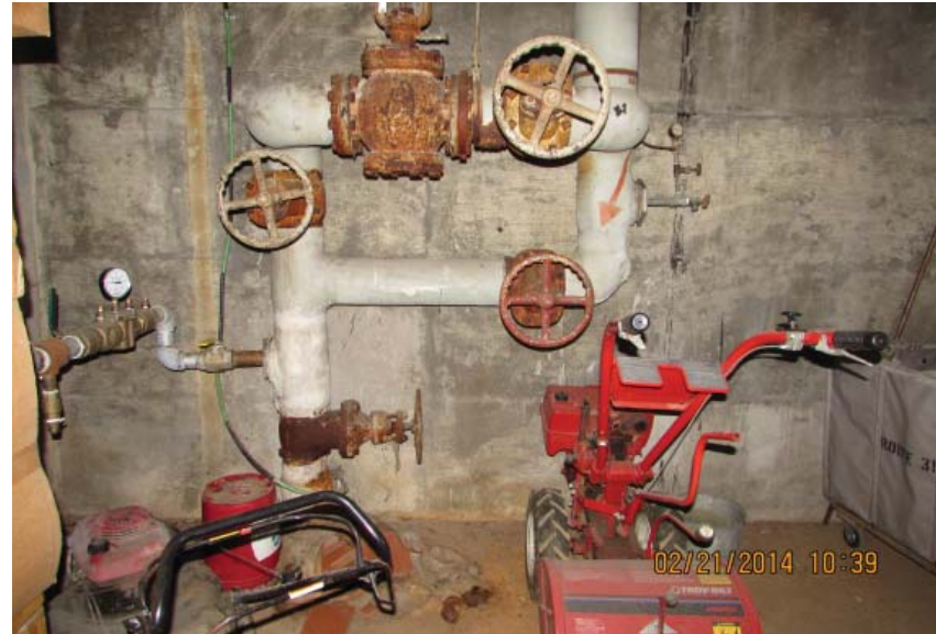
Incoming Water Service - Main Building
