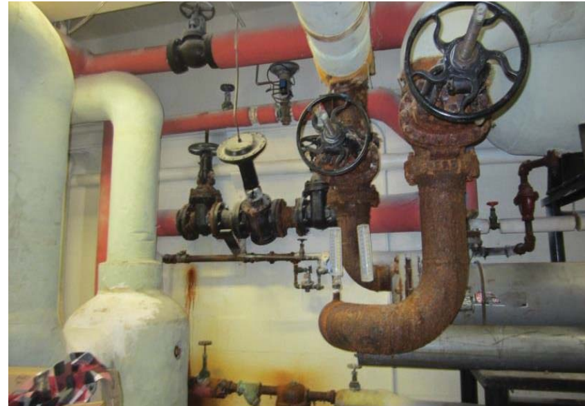
Steam-to-Hot Water Converter – Corroded Piping and Valves
