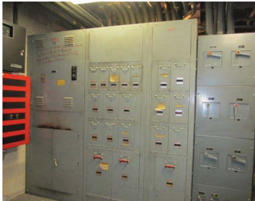
Original 208Y120 volt switchboard
