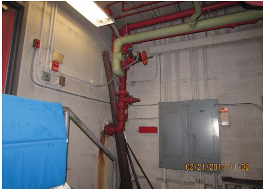
Incoming Water Service - Main Building
