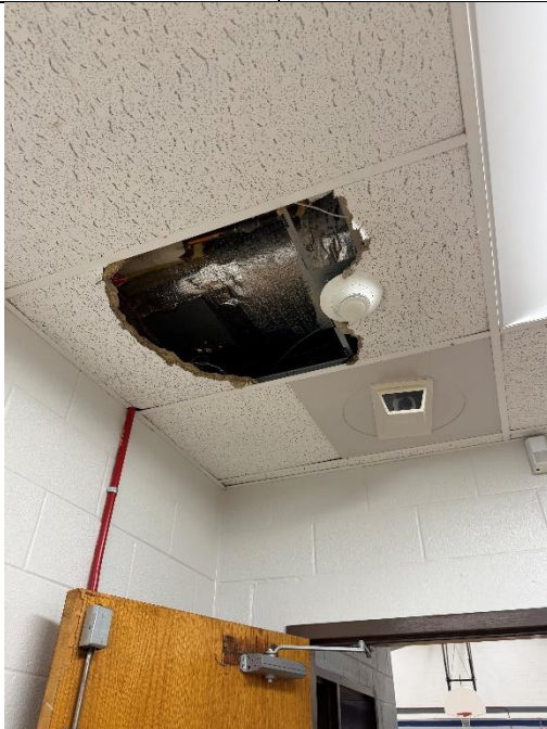
Image 3 Outside Gym Entrance Missing ceiling tile.
